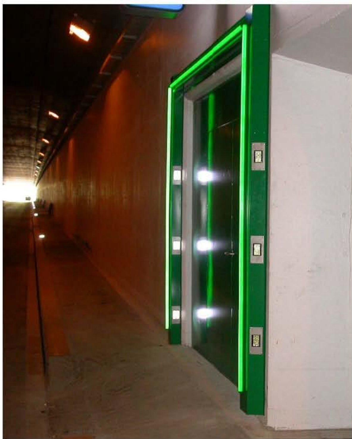
Emergency exit in road tunnel
